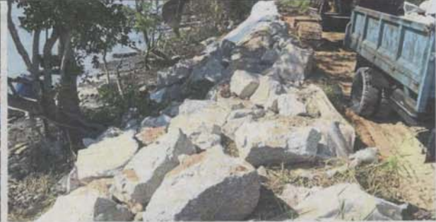
Last year, the bunds at Sungai Lang in Sabak Bernam were reinforced by the state Drainage and Irrigation Department. — Filepic
